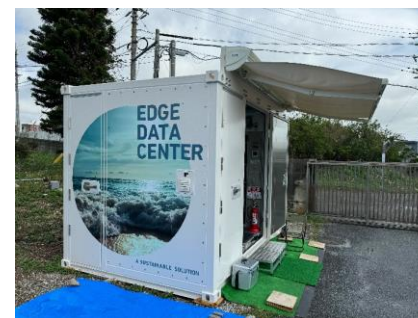
Container Data center at KDDI site in Okinawa
